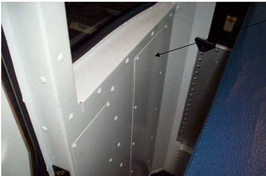
This panel and same panel on opposite side of emergency door are to be inspected for adhesive
